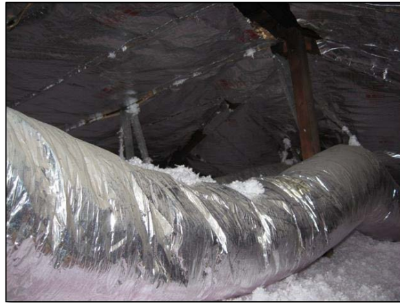
Figure 4.24. Radiant barrier installed on rafters, ridge vent, and additional blown-in insulation installed.
