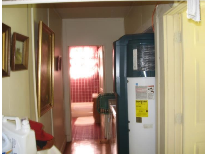
Figure 4.13. Hybrid heat pump water heater.
