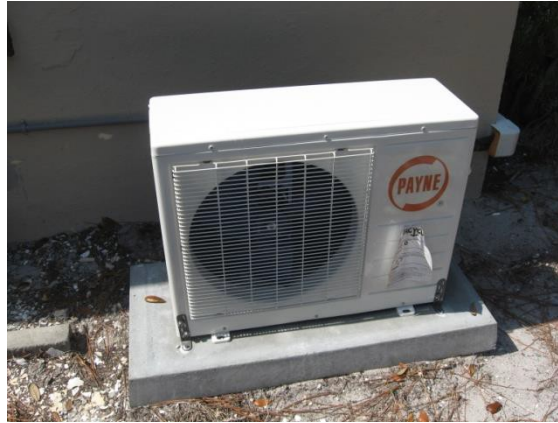
Figure 4.25. Outdoor mini-split unit mounted on a hurricane-rated pad.
