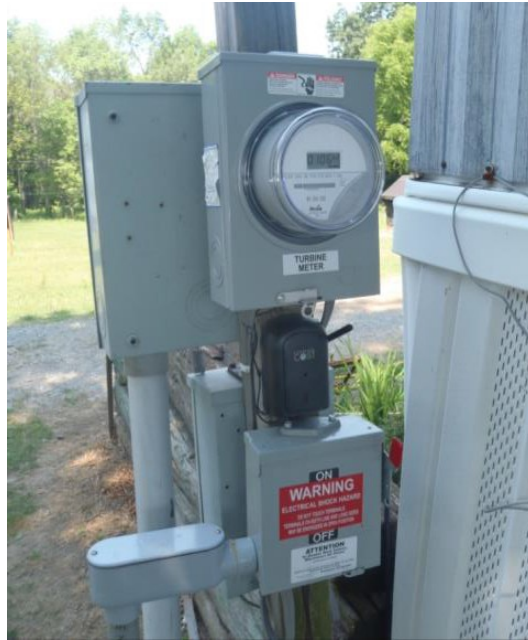
Figure 4.19. Electric meter connected to a wind turbine.
