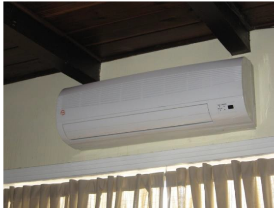
Figure 4.26. Indoor mini-split unit mounted above windows to condition the living room, kitchen, and rear rooms.
