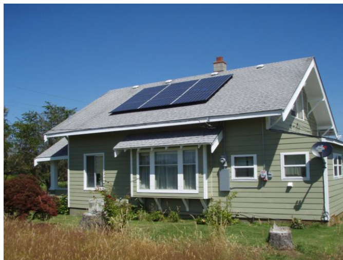
Figure 4.2. Solar PV panel installation.
