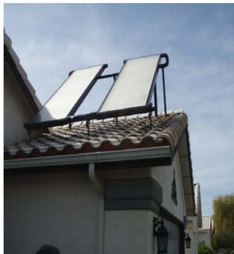
Figure 4.5. Solar water heater collectors.
