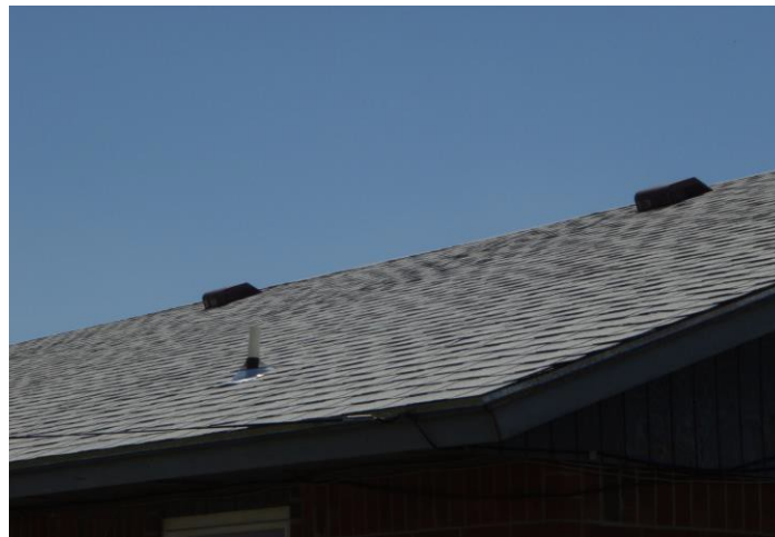
Figure 4.21. Example of a cool roof.
