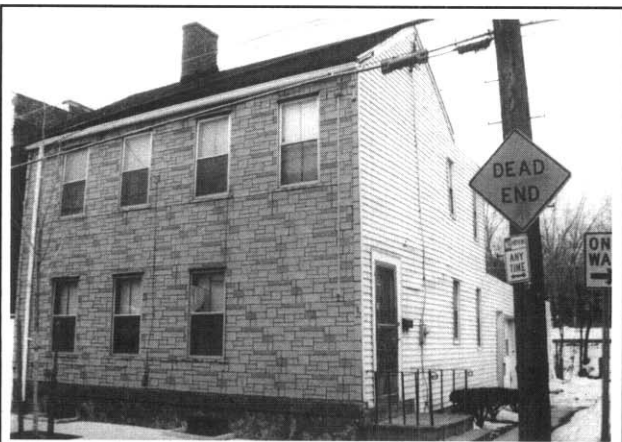
Retrofit siding hides major holes that cause air leakage.
