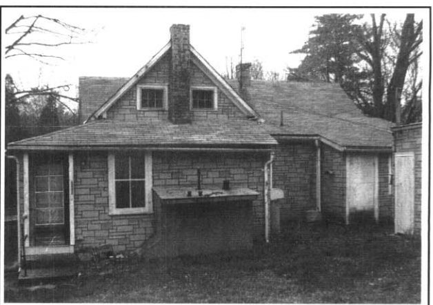
Built in sections over many years, this dwelling has major leaks between the main house and newer additions.
