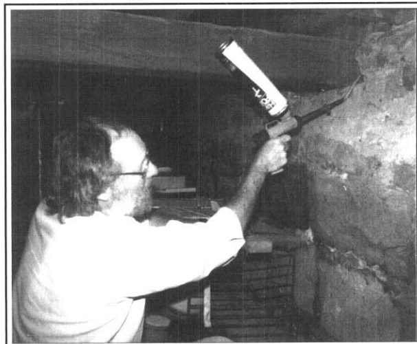
Air sealing at sill plate with foam. This infiltration-stopping measure is necessary with most weatherization jobs.
