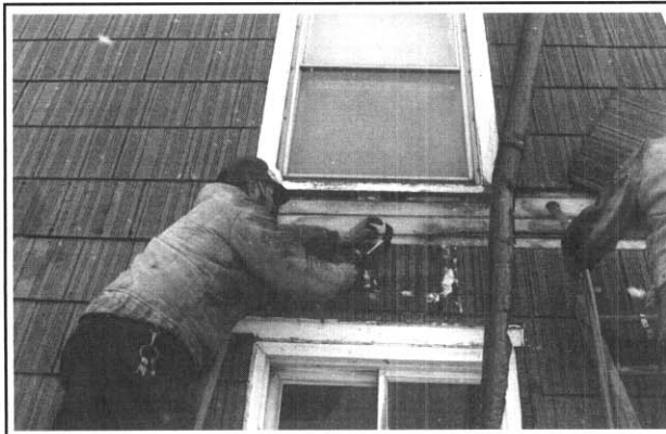
Preparation, insulation, and cleanup keeps two weatherization team members working for most of a day.
