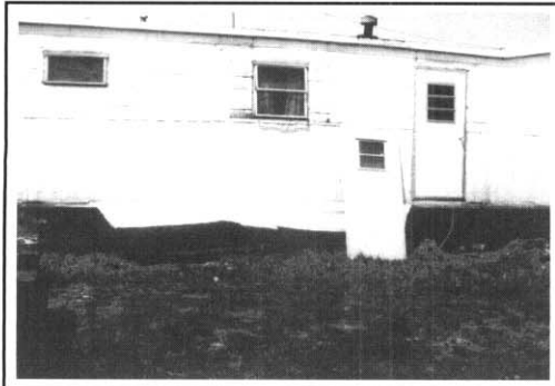
New doors and windows sometimes save energy, but air sealing ducts in mobile homes are usually a more cost-effective retrofit.
