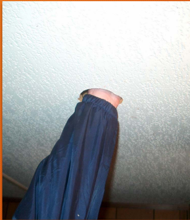
This hole should be in a closet
