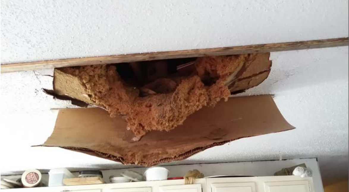
Figure 30. Ceiling damage from roof leaks.
