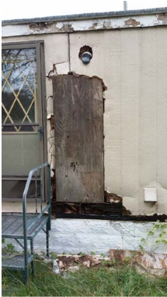
Figure 31. Example of deteriorated exterior.
