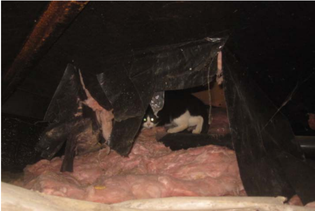
Figure 32. Tight skirting is needed to keep animals out of the belly area, where they can otherwise do significant damage to insulation.
