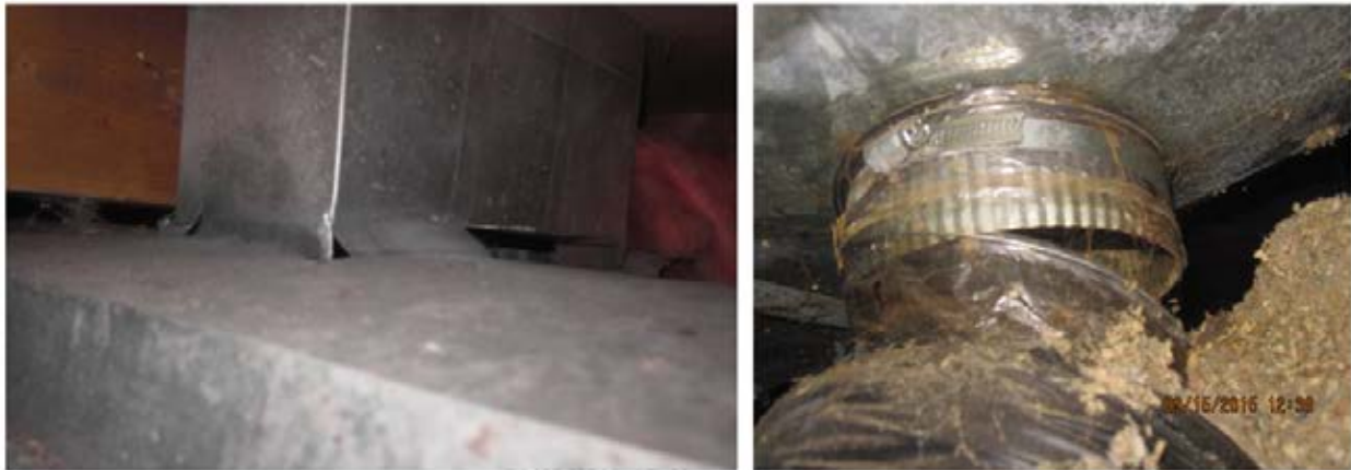
Figure 23. Example of duct leaks.
