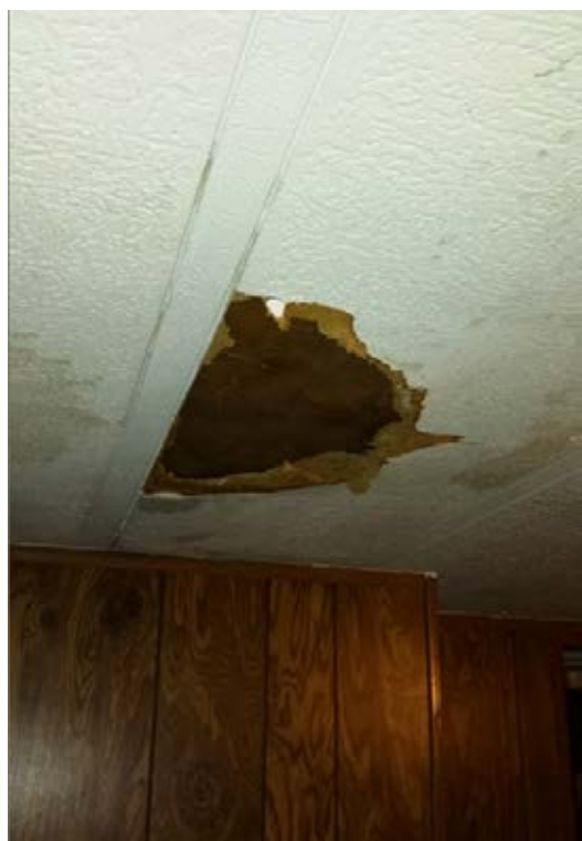
Figure 28. Deteriorated ceiling area. These are often due to water damage.
