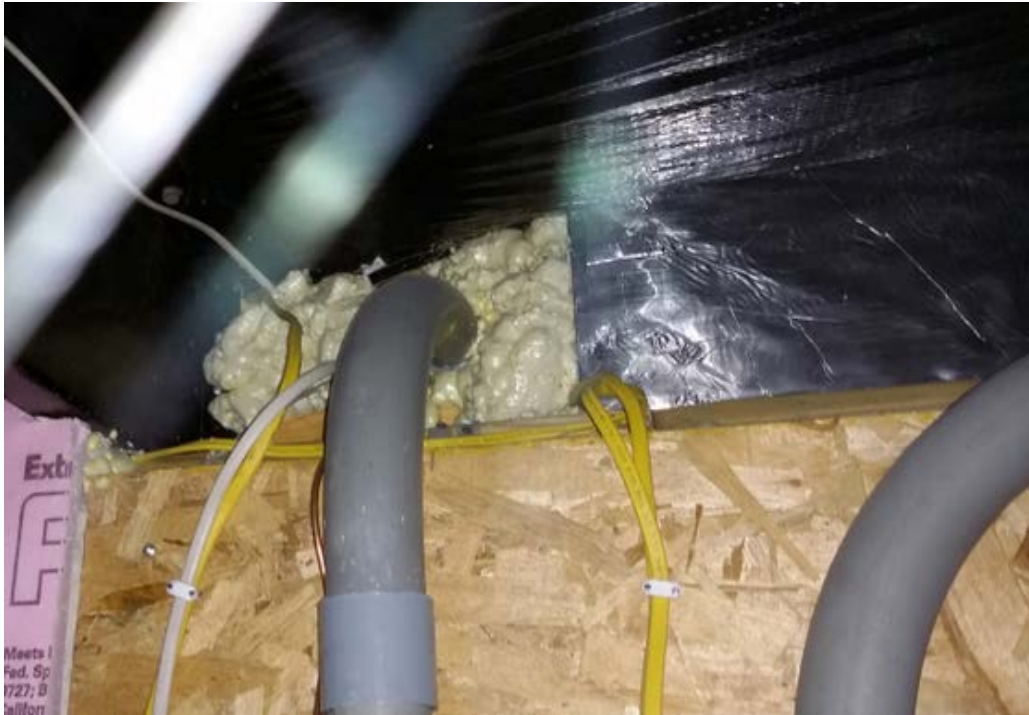
Figure 21. Evidence of air sealing of electrical penetrations by local weatherization agency in a site-visit home.
