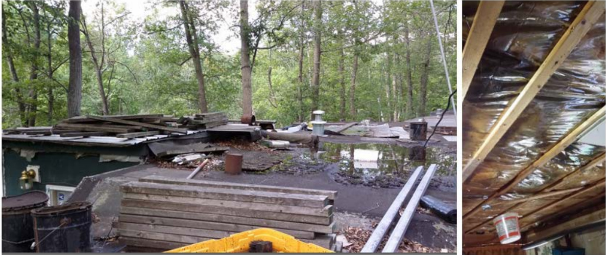
Figure 29. This manufactured home has standing water on its flat roof, and a large section of fallen ceiling.
