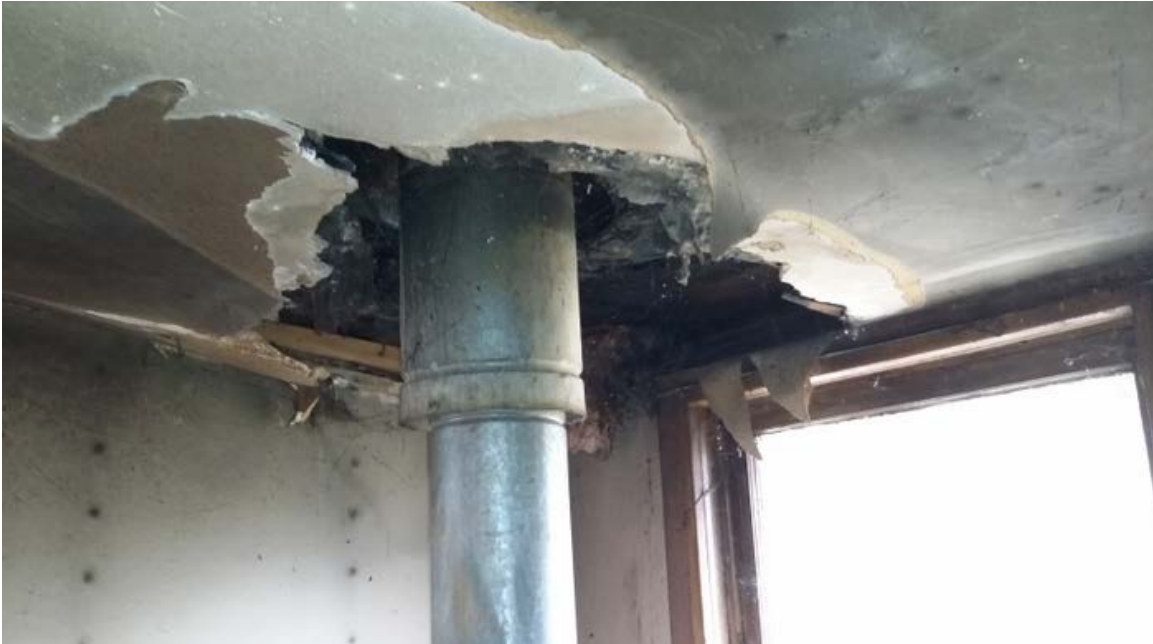
Figure 37. Fire damage from a wood-burning stove in a manufactured-home addition.
