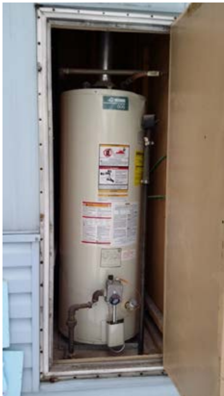
Figure 24. Example of a water heater in an exterior closet.
