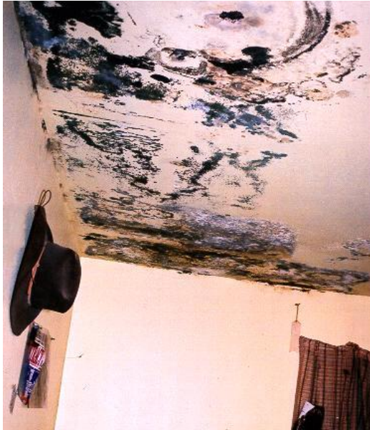
Figure 3.4. Water damaged ceiling due to a leaking roof.
