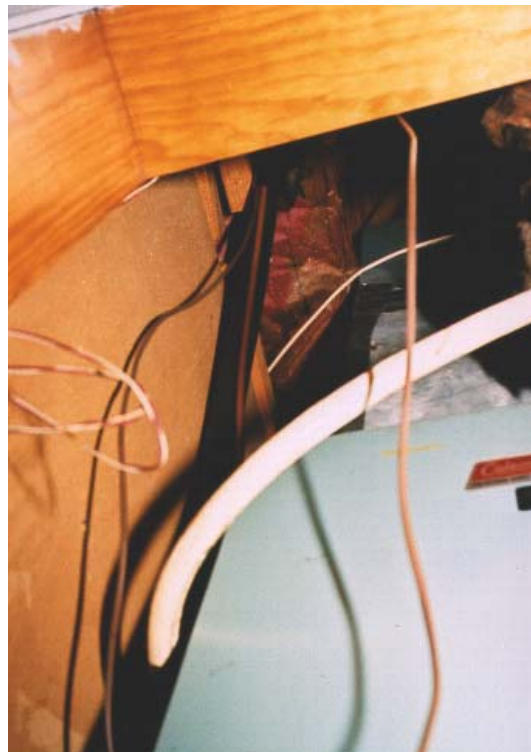
Figure 3.2. Unsealed equipment chase permits infiltration.
