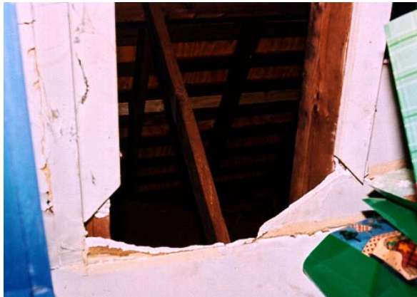
Figure 3.1. Broken attic access hatch allows a high infiltration rate.
